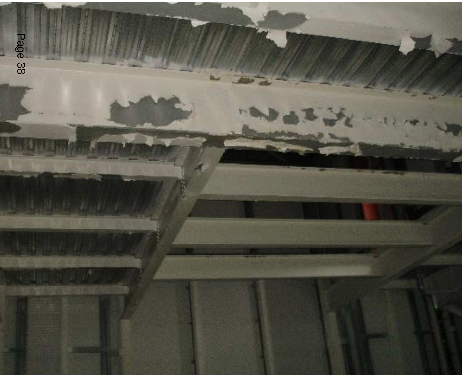
Defective paintwork on interior steel frame
